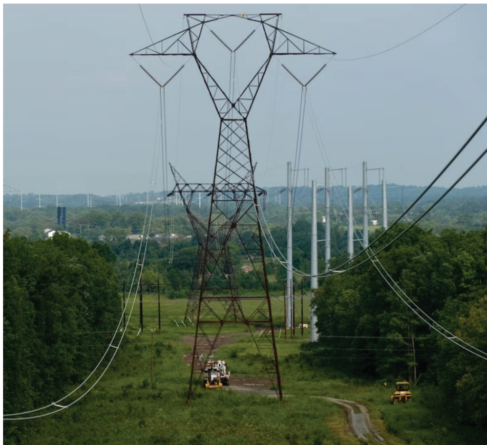
Data Centers/Power lines Dominating the Landscape and Neighborhoods. Photo credit: Washington Post/Xiaomei Chen
