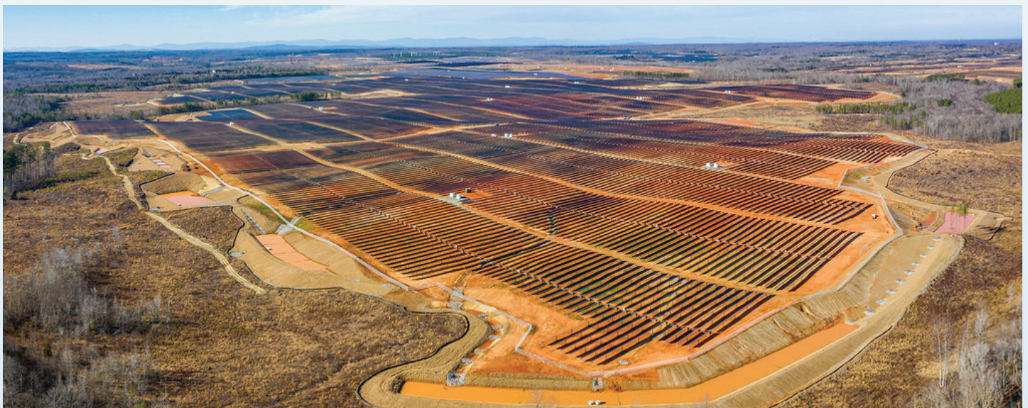
Solar facility under construction in Spotsylvania County. Photo Credit: Hugh Kenney, Piedmont Environmental Council
